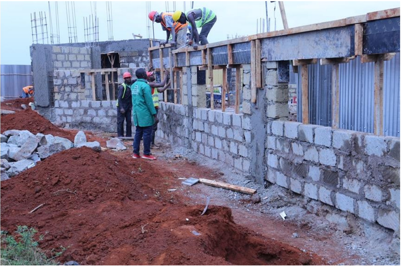
ABOVE: September 2019 status as the gate is erected with skill and precision at Amani Ridge | The Place of Peace
