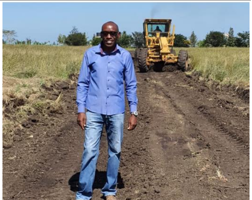
ABOVE: Mr. Charles Muraguri, the Director of Projects at Optiven Group during the kickstarting of the roads construction at Victory Gardens | Kitengela Phase V
