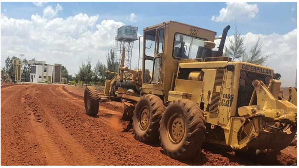
ABOVE: Heavy machinery at work inside AMANI RIDGE | The Place of Peace to ensure the infrastructure of the road networks is done within the required standards.
