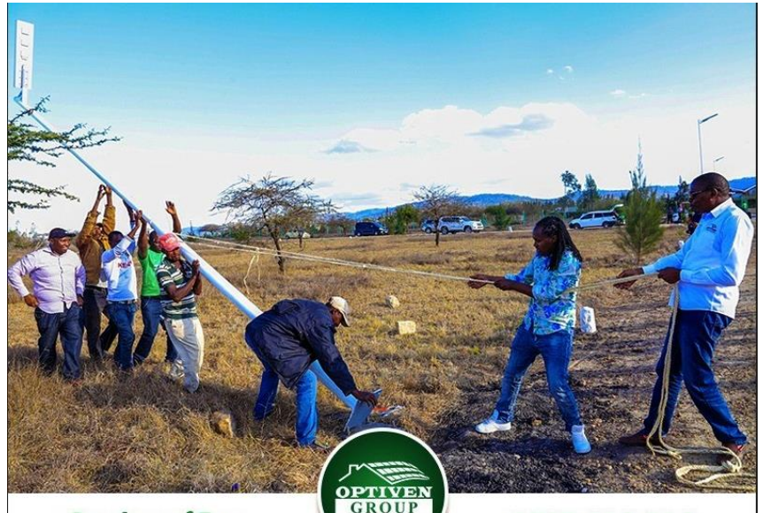
ABOVE: Mr. George Wachiuri, Optiven Group CEO, ( far left ) joins the team of Engineers during the installation of street lights at the Garden of Joy in Machakos in October 2020
