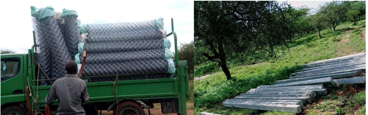
ABOVE: Materials arrive to add value at Love Gardens by Optiven in Kajiado County on 25 th February 2021
