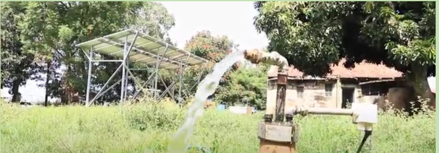
ABOVE: Water & solar installed at Winners Gardens with the project dotted with mature fruit trees
