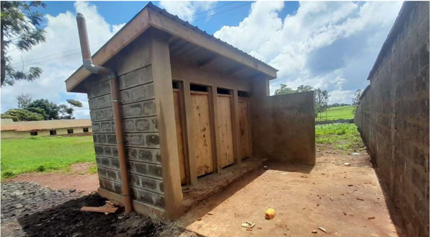
ABOVE: The toilet block donated by Optiven through its Go Green Initiative under construction at Kiama Primary School on 18th November 2023
